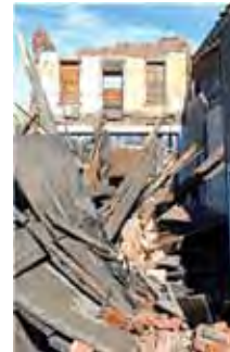
Moderate earthquakes can cause devastating damage to older masonry buildings. This photo shows a roof fall that occurred during the 2008 M 6.0 earthquake in Wells, Nevada. Earthquakes of this magnitude can occur anywhere in Idaho. (NBMG photo.)
