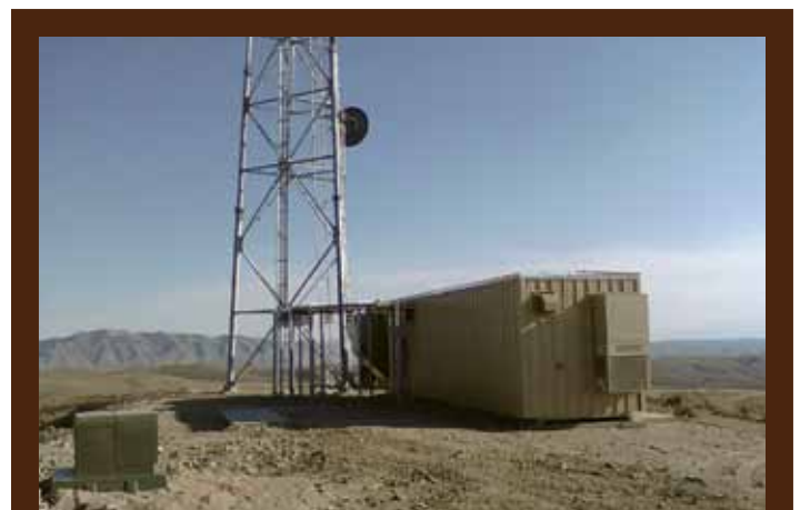
The Hell Hole project is in the final stages and should be completed by the spring of 2012.
