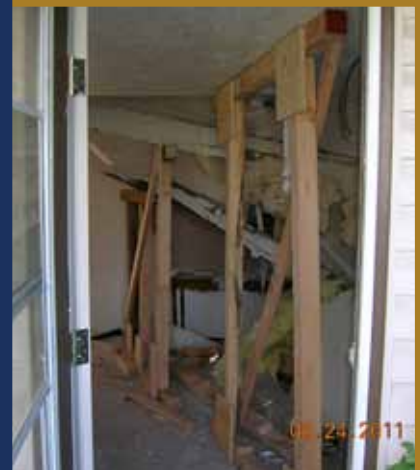
Here you can see some of the "T" shoring that was done by the technical rescue personnel to make the structure safe to enter for the rescue attempt.
