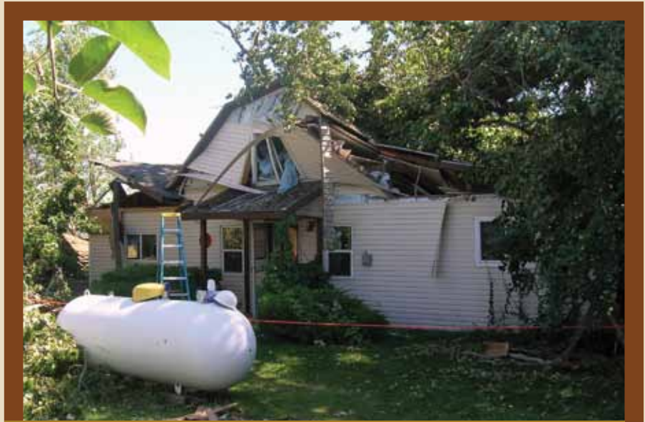
A large popular tree, approximately 26 feet in circumference, crashed into this residence and crushed one of the occupants.
