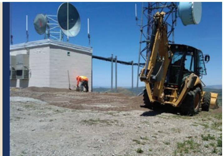
PSC completed several fire mitigation projects this summer, like this one at Chinese Peak, to prevent damage from wildfires.
