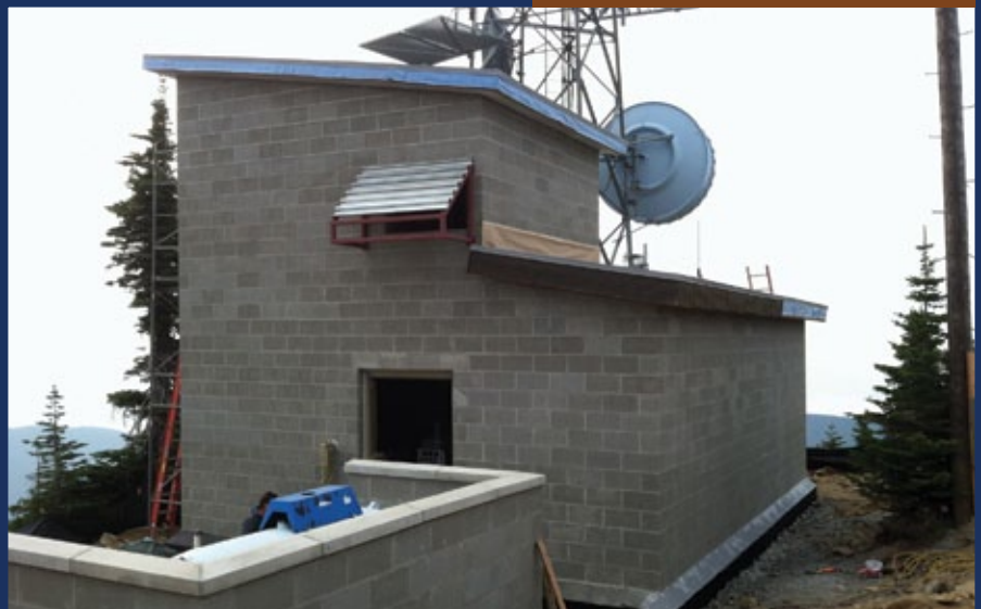
The new facility on Schweitzer Peak provides upper level access for better winter ingress as well as better overall functionality.
