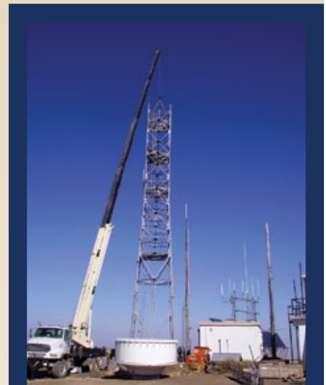
On Bennett Mountain, in Elmore County, PSC removed the existing tower and constructed a new 100 foot, self-supporting tower.
