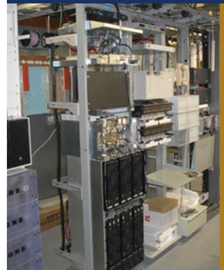
Example of a Trunked Radio Installation.
