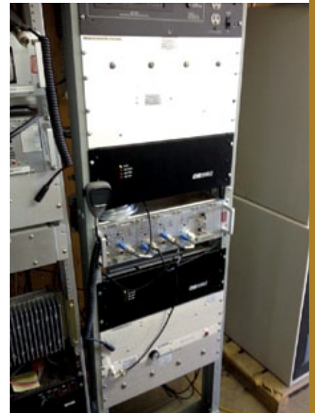
Example of a Conventional Radio Installation.
